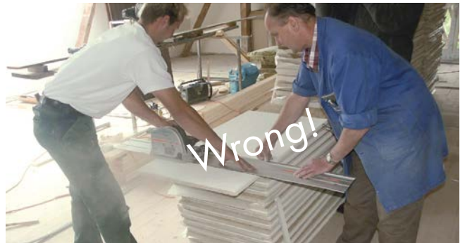
Not like this! Never cut acoustic tiles on a pile!
