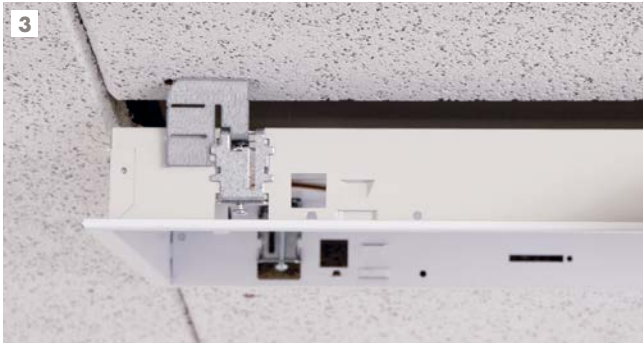
3 Hang the ceiling light. Fix with the supplied side wings to the T-profiles, CD profiles or wooden battens. Adjust the installation height of the light to the existing suspension height.
