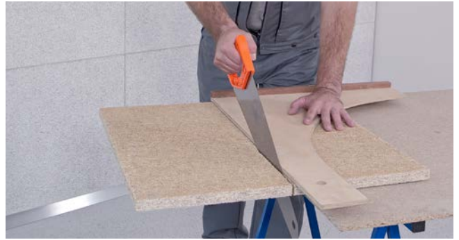
Jack saw Lay the acoustic tile down face side up. Always work with a guide. Support the free end of the tile.
