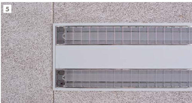
5 Installed modular light. The tile joint is covered by the frame.
