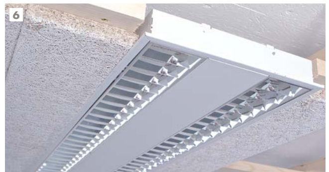
6 The joint between the HERADESIGN® acoustic tile and the light is covered by the frame.
