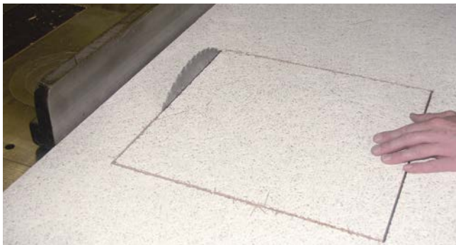
Cutting out of the opening/cover tile from the reverse side of the tile.
