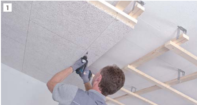
1 Exchanging the ceiling grid for the installation of modular lighting: Additional cross profiles and hangers required in the area of the exchange.
