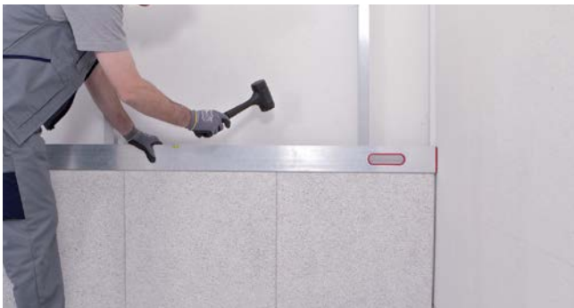
Align the tiles and the main profile before fixing it with the self-drilling screws.
