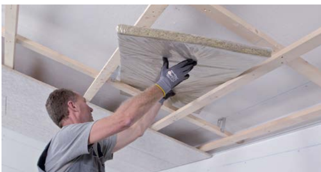
Insert HERADESIGN® acoustic overlays or other acoustic overlays, step-by-step when installing the HERADESIGN® acoustic tiles. Absorber tiles that are pushed between the wooden battens are cut to size.
